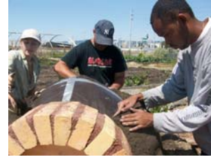
Allen Beene, the GYP OJT, helping to put the finishing touches on the newly built farm earth oven.
